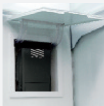
Air purification system.
